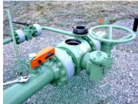
Argus 4" Pig Receiving Valve with gear operator and Hi-T Pigalert pig detector.
